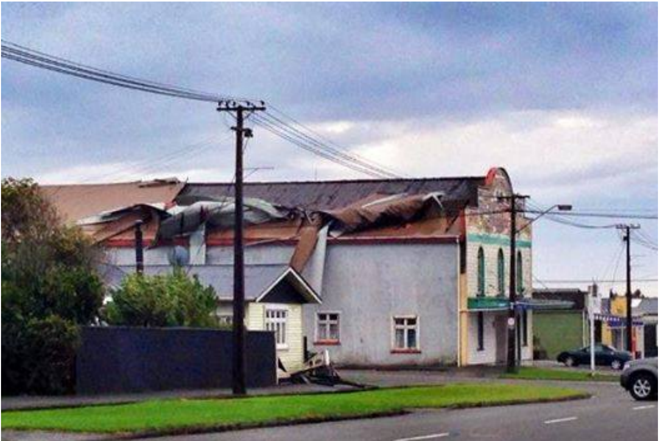
The Runanga Miners' Hall after Cyclone Ita blew through in April 2014.
